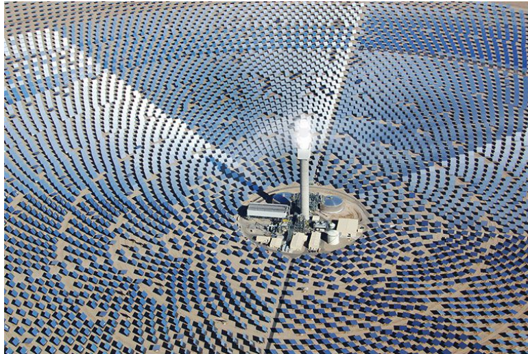
Figure 6: Use of molten salt in a concentrated solar power system, where the molten salt is circulated through the power tower in the middle, stored in insulated tanks (Solar Reserve, 2017).
