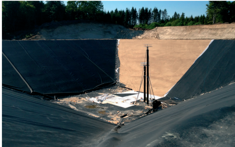
Figure 5: Construction of Dronninglund pit storage for solar heated district heating system (PlanEnergi, 2016).
