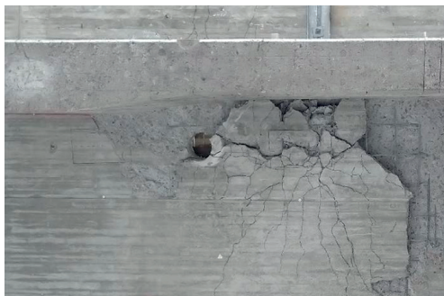
Figure 34. The Kiruna Bridge at shear and punching failure of the deck slab, view from below (Image by Niklas Bagege).
