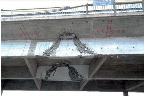
Figure 33. The Kiruna Bridge after shear failure of the girders (Image by Niklas Bagge).
