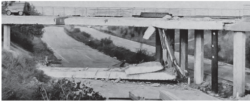
Figure 20. The Brønsholm Bridge after collapse (Pedersen et al. 1980).
