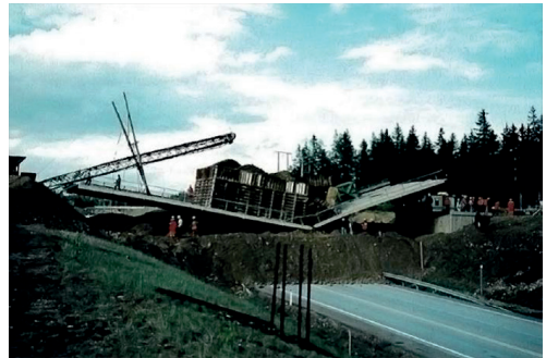
Figure 27. The Smedstua Bridge at collapse (Statens Vegvesen 1998).
