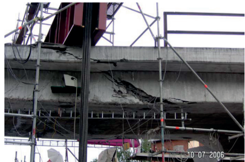
Figure 31. The Örnsköldsvik Bridge after failure of the trough girder (Image by Lennart Elfgrén).
