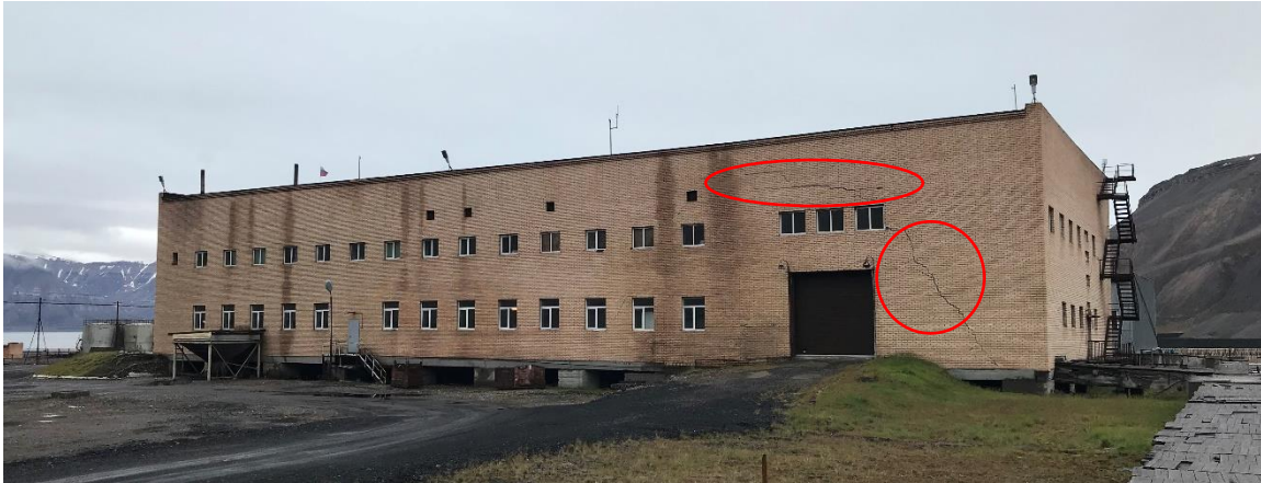
Figure 18. Cracks (highlighted with red circles) on the north-facing wall of the multi-purpose garage in Pyramiden.
