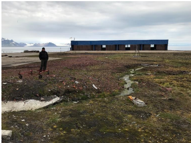
Figure 17. Drainage coming from under the building "Komplex GRZ" in Barentsburg (continuation, building is behind the photographer).
