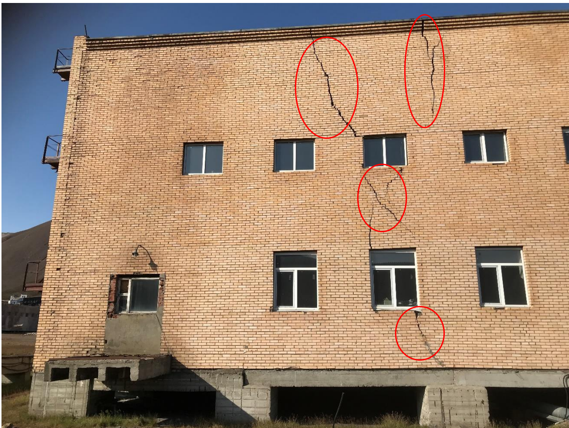
Figure 19. Cracks (highlighted with red circles) on the south-facing wall of the multi-purpose garage in Pyramiden.
