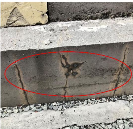
Figure 22. Cracks (highlighted with red circles) on foundation of the “Magnetittlageret” garage.
