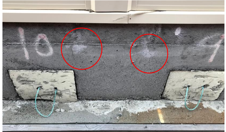
Figure 21. Cracks (highlighted with red circles) on foundation of the “Magnetittlageret” garage.
