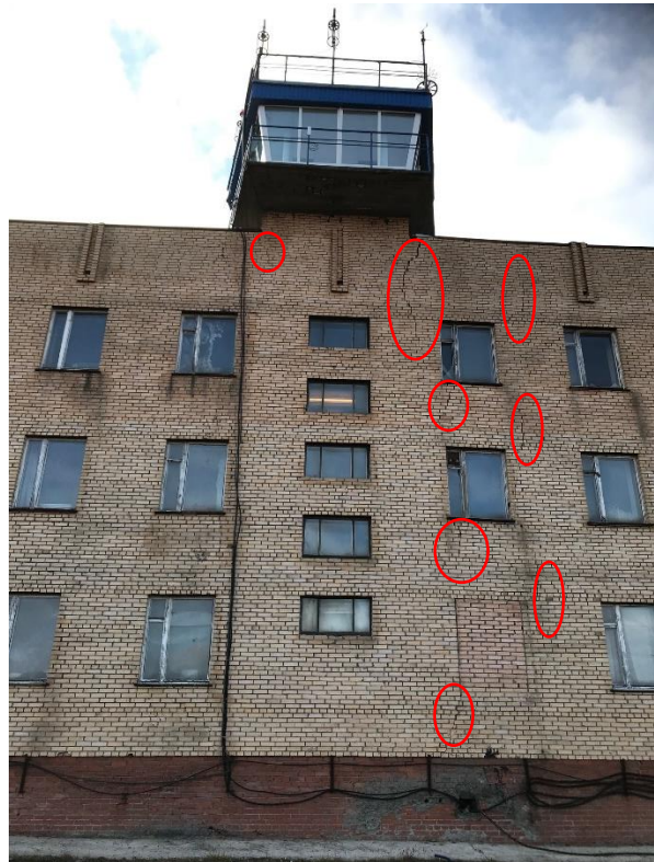
Figure 15. Cracks (highlighted with red circles) on the east-facing wall of the building "Komplex GRZ" in Barentsburg.
