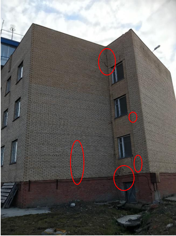
Figure 14. Cracks (highlighted with red circle) on the north-facing wall of the building "Komplex GRZ" in Barentsburg.
