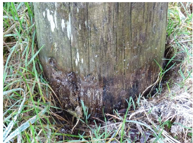
Figure 2: Rot in a pole (DG=4)
