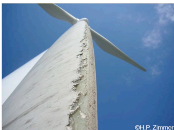
Image 1: Leading edge erosion ( http://www.hogrehojder.se/vindkraft.html )
