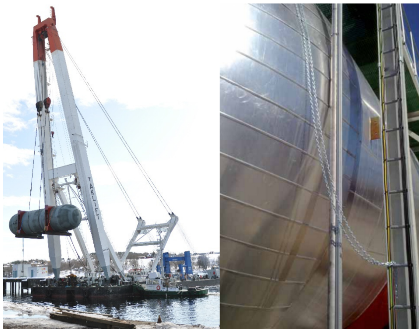
Figure 4: Steam accumulator installed in Sarpsborg (NO) – Photos: Borregaard AS / Sarpsborg Avfallsenergi AS.
