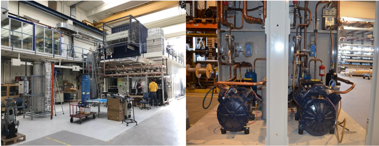
Figure 19: Some of the equipment installed in the HighEFF Lab: CO 2 heat pump facility (left) and propane & butane compressors (right).
