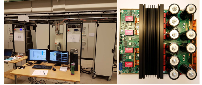
Fig. 6. Overview of MMCs and view of a converter cell
