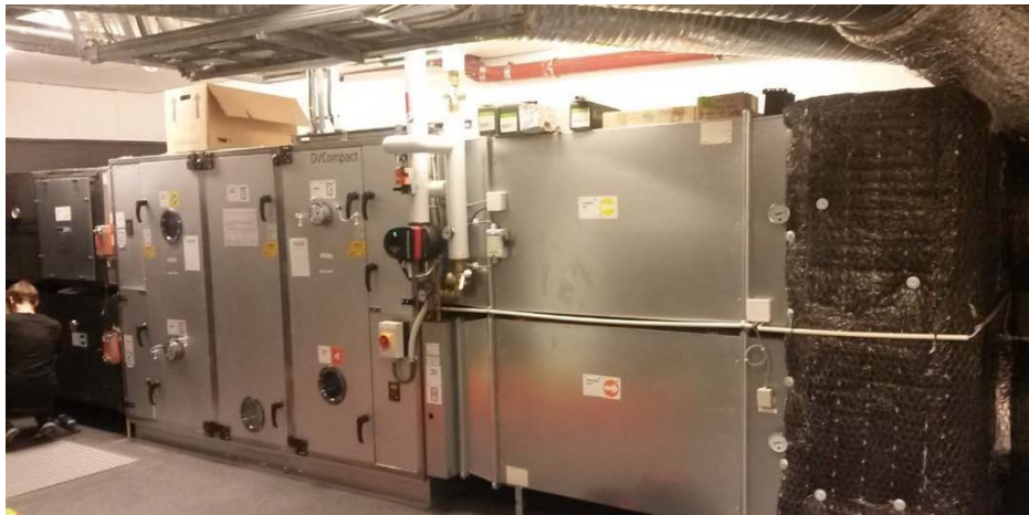
Figure 31 Picture of the air handling unit at Øya kindergarten.
