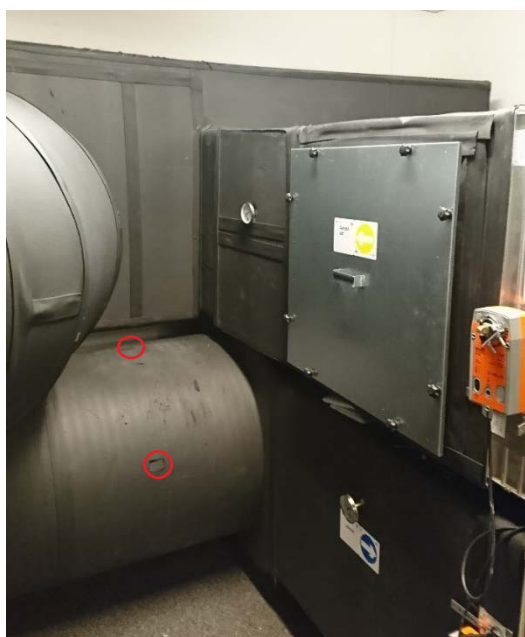
Figure 33 Picture of the air intake and exhaust duct from one of the AHUs at Øya kindergarten. Red circles indicate where the holes for measurements with the velocity traverse method are located.
