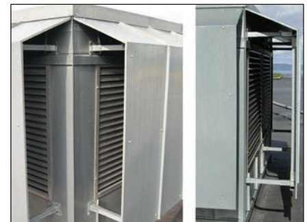
Photo 5: Shielded fresh air ventilation intakes. Note that it is also recommended to shield the open sides shown here, i.e., the only air intake is from under the shielding and upwards.
