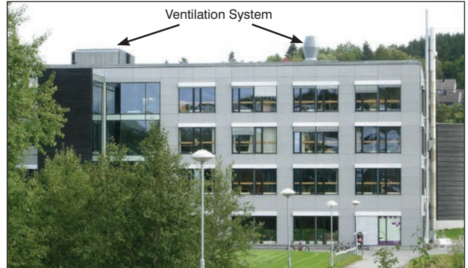
Photo 1: University campus building with fresh air ventilation intakes on roof with previous snow and rain inlet problems.
