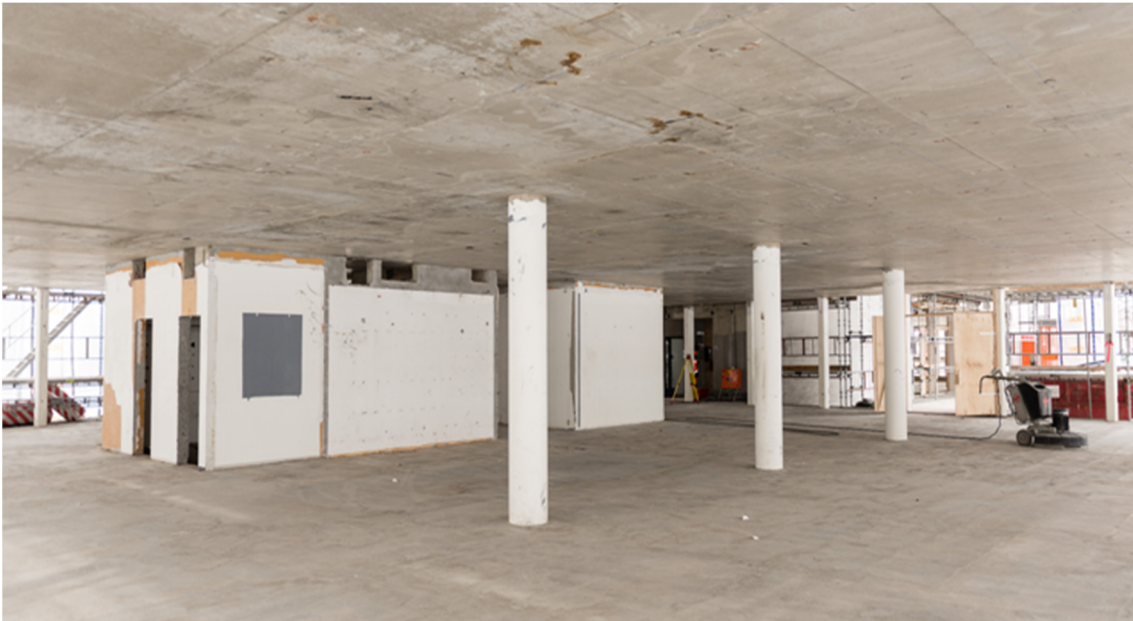
Figure 8.5 The Construction process at Powerhouse Kjørbo, keeping the existing steel and concrete substructure. Photo: Snøhetta
