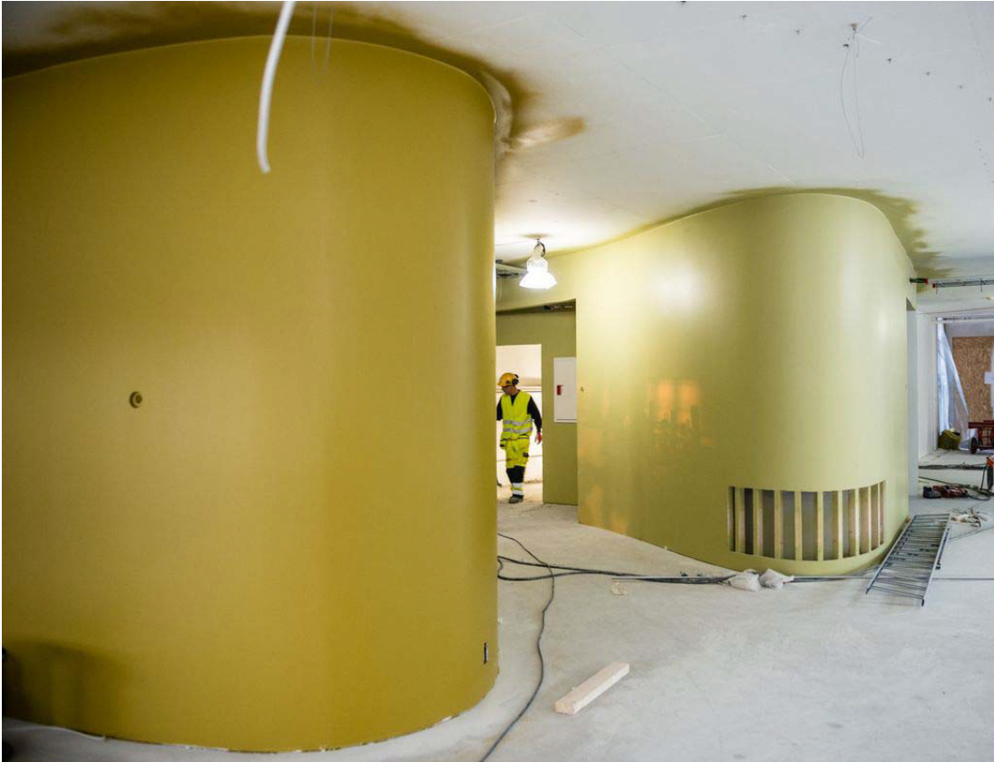
Figure 8.6 The Construction process at Powerhouse Kjørbo; interior shafts for ventilation. Photo: Snøhetta
