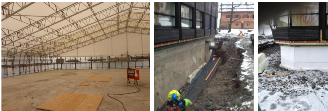
Figure 2.7 The roof of Powerhouse Kjørbo prepared for improved insulation (left), and work on improving the insulation on the external wall (right). Photos from Jenssen (2016).
