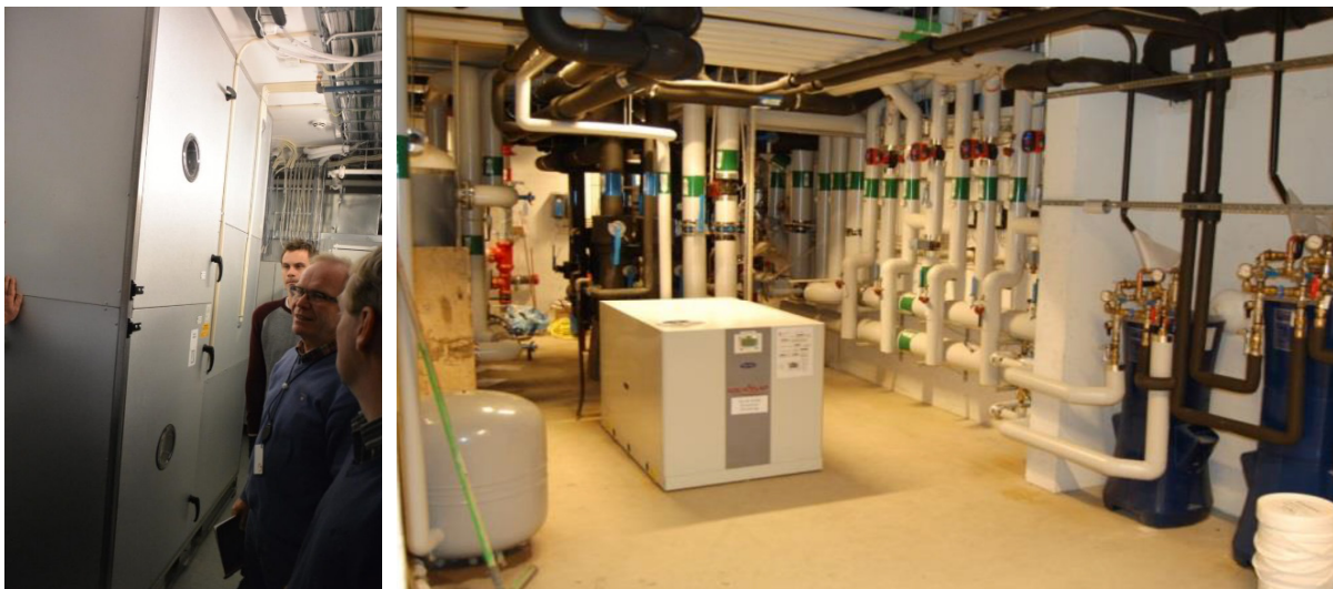
Figure 5.1 The technical room at Powerhouse Kjørbo. Photo: Asplan Viak.
