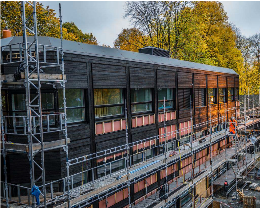
Figure 8.7 The Construction process at Powerhouse Kjørbo; fitting of wood cladding. Photo: Snøhetta
