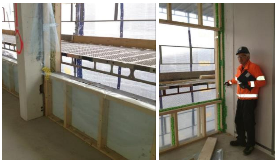
Figure 2.9 Thermal insulation on external walls of Powerhouse Kjørbo Block 5 (left), and sealing around windows (right). Photos from Jenssen (2016).
