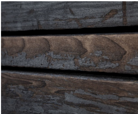
Figure 2.16 Charred wood in the façade. Photo: Snøhetta.
