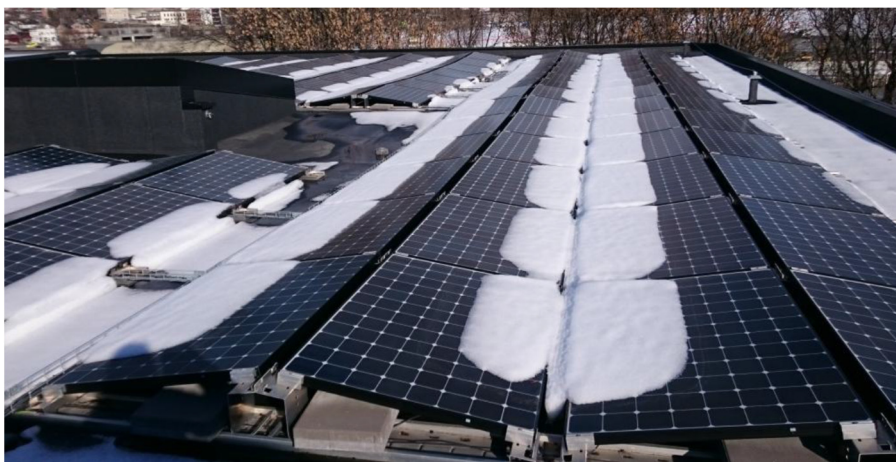
Figure 4.15 The roof of Block 4 from March 10th, with snow on the modules. Photo: L. Ødegården.
