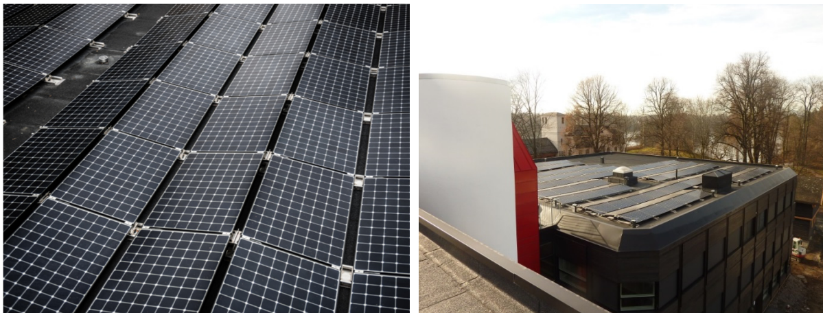
Figure 4.14 Photos showing the placement of the PV panels on the roof. Photo: Skanska.
