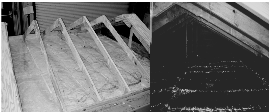
Fig.5. The tested attic construction [left] with only the fibreglass batts between wooden beams and without roof shelter and [right] a view in the attic construction when the GFPs with the attic radiant barrier are installed (Yarbrough et al. 2007).
