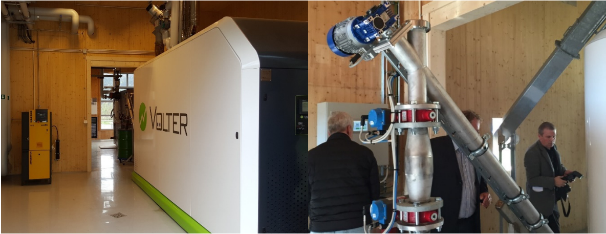
Figure 5.4 CHP unit at Campus Evenstad, photo courtesy of ETA Norge AS.
