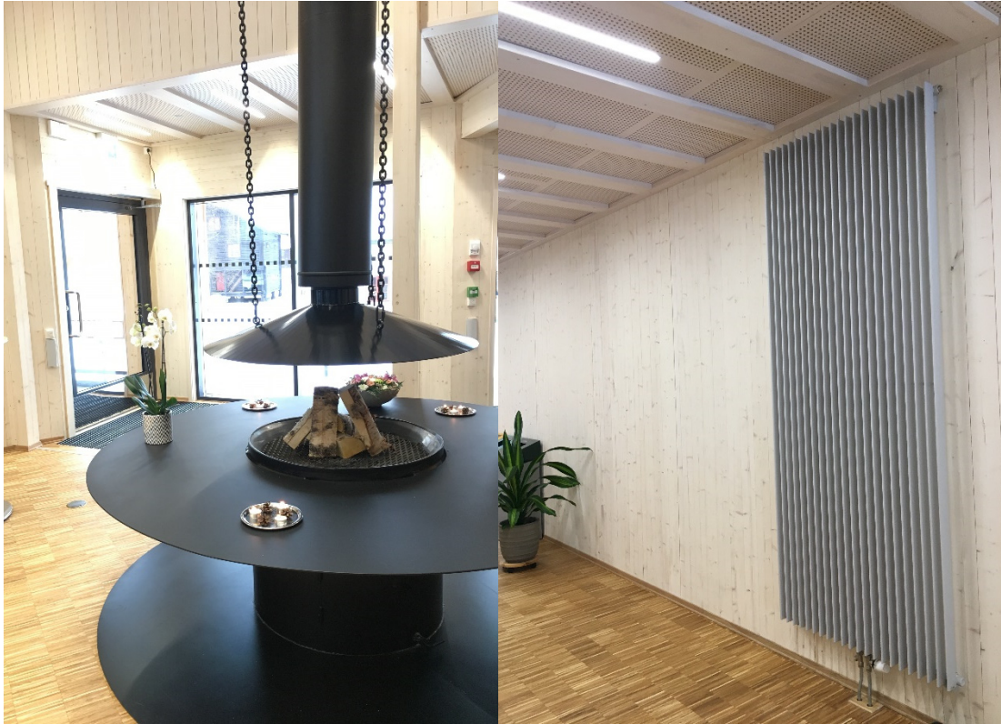
Figure 5.2 Photographs of the wood-burning fireplace and wall mounted radiator. SINTEF.
