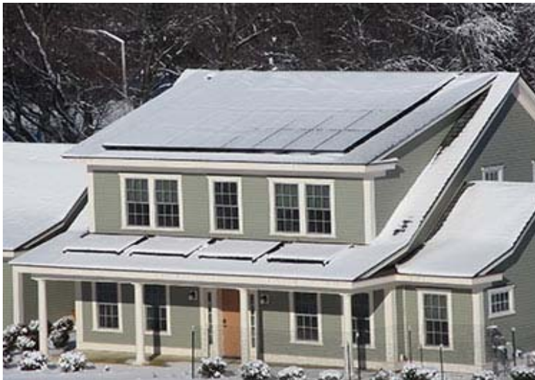
Figure 9: Snow on photovoltaic modules mounted on pitched roofs. Note that snow might slide off one roof and fall onto the other, possibly damaging the panels mounted on it (NIST 2014).
