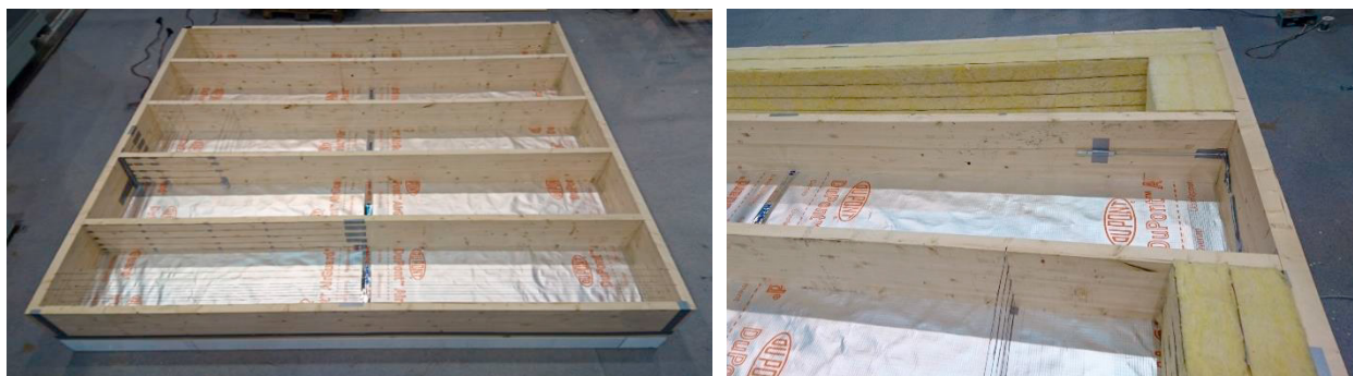
Fig. 1. Photo showing the timber frame test section under construction with a reflective foil at the hot side of the cavities and thermocouples mounted for measuring temperatures inside the cavities. Edge insulation partly mounted, (right).
