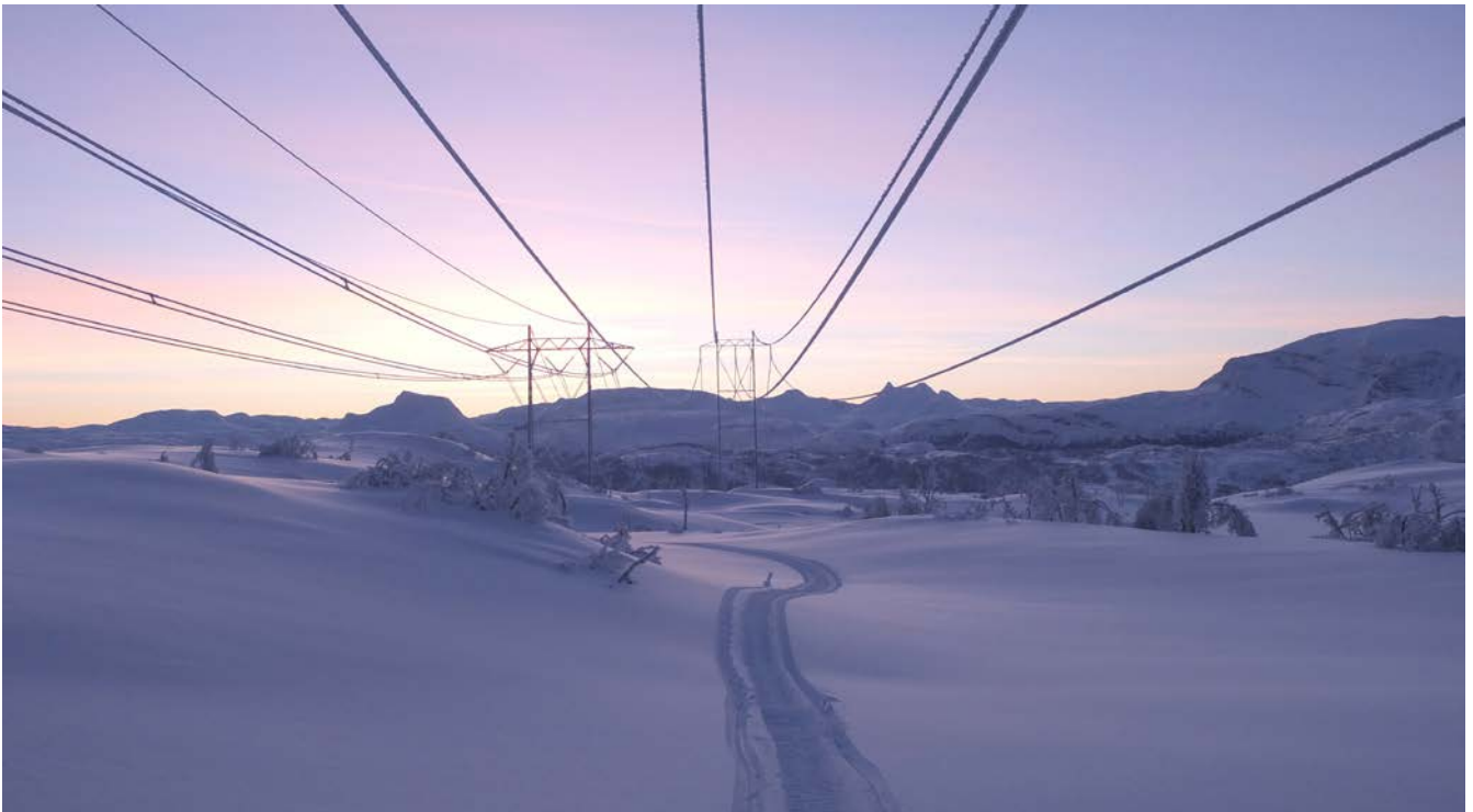
Conflicts often arise when new power lines are planned and constructed. Studies carried out by CEDREN show that disagreements can be avoided or significantly reduced. Photo: Statnett
