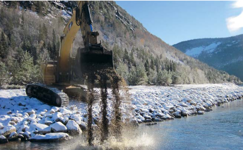
Once a diagnosis has been established practical measures may be undertaken in accordance with detailed descriptions in the handbook. Here, a new spawning area is under construction. Photo: Ulrich Pulg.
