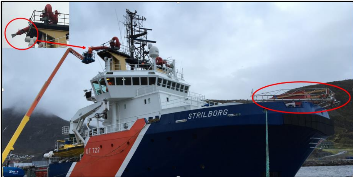
Figure 5-6 Installation of prototype systems on MS Strilborg at Hammerfest, May 23-25, 2016). Upper left: Deflector on Fi-Fi-monitors. Right: Container based high-capacity water-flow boom and high / low dispersant (manifolds) at the bow. Part of the "Oljevern 2015 program "Mechanical Dispersion of Thin oil films" funded by NOFO.
