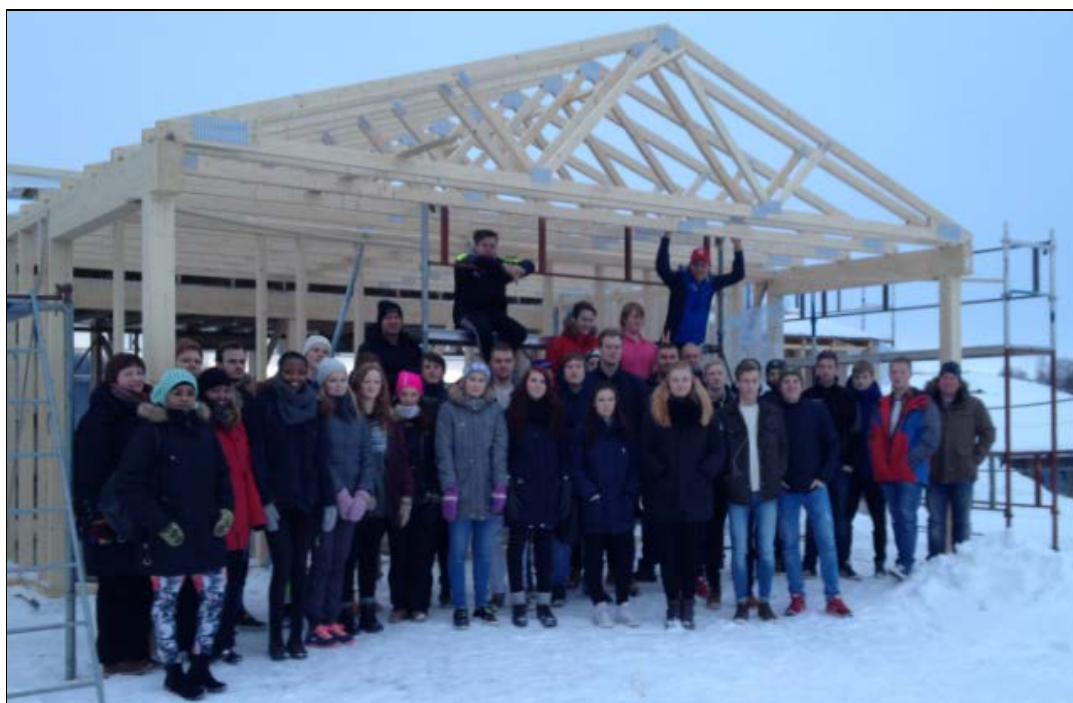
Figure 1: Pupils and teachers from Building Studies and Health Care Studies on the building site in Overhalla, January 2015
