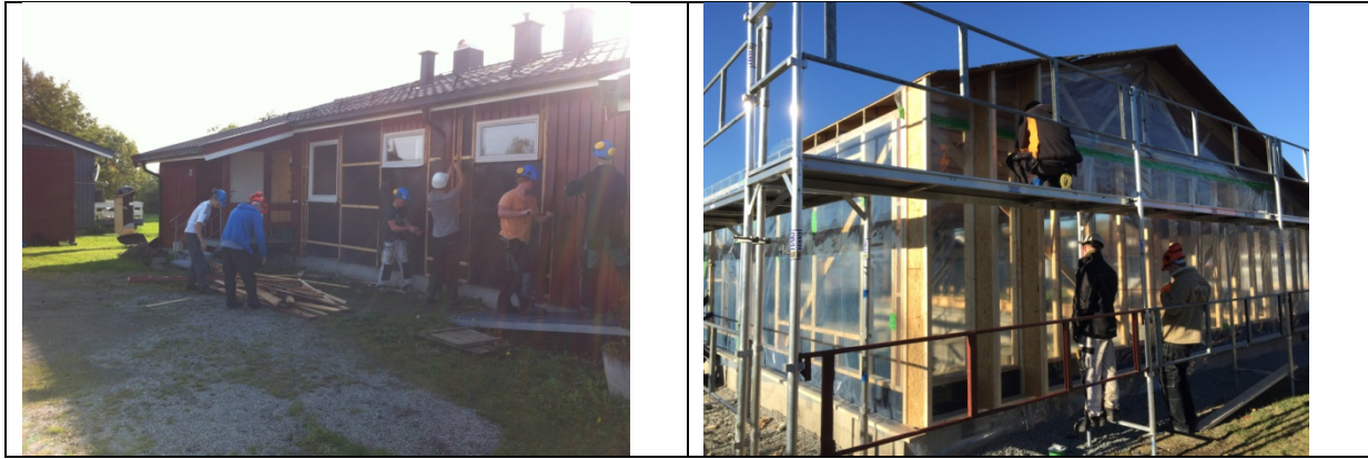
Figure 3: Left: Demolition of the wall construction. Right: Construction of the new retrofitted wall construction.
