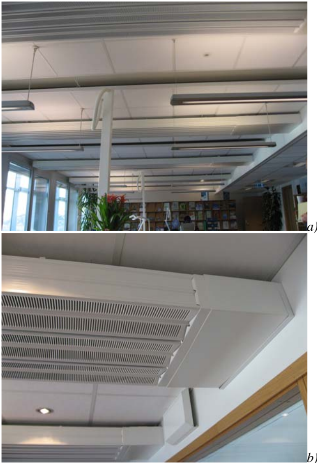
Figure C-10. Integrated ventilation and cooling in the ceiling elements, a) overview b) detail (photo Sintef Byggforsk / Matthias Haase)
