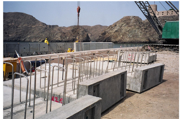
Figure 7-2: New precast concrete seawall elements to replace an existing seawall adopting SSR (1.4462)
