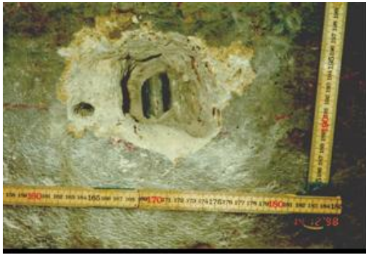
Figure 1-5: Typical picture of breakout exposing non-corroding SSR /1/
