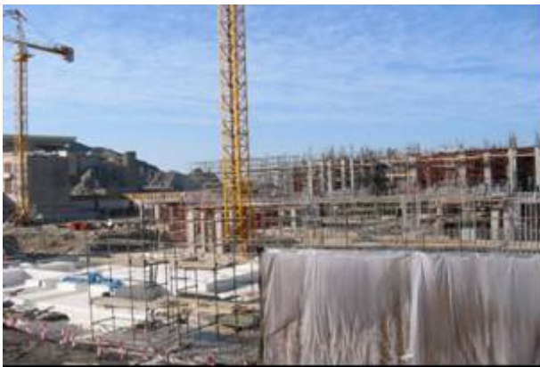
Figure 7-1: A large building complex under construction in the Gulf directly facing the sea
