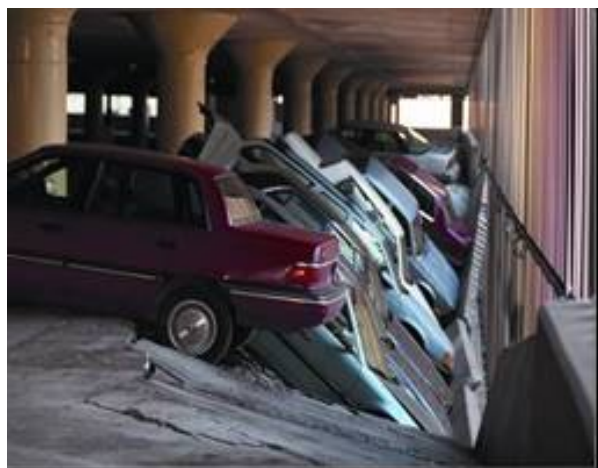
Figure 1-2: Corrosion damage in car park deck
