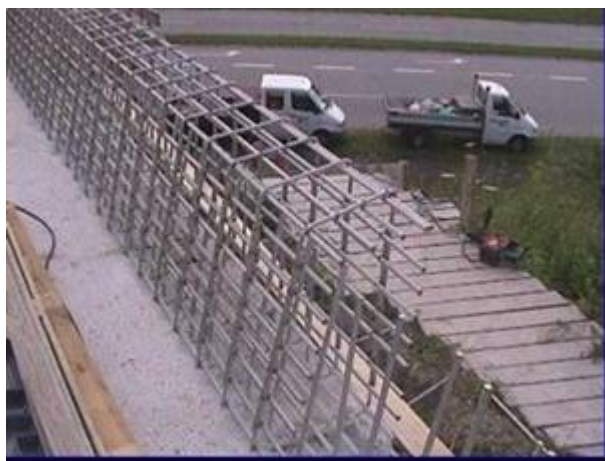
Figure 7-6: Replacing edge beams and parapets on bridges in Denmark exposed to de-icing salt.
