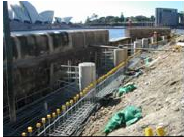
Figure 7-5: Reconstruction of the seawall in Sydney Harbour using SSR (1.4462) following extensive corrosion damage of the reinforcement.
