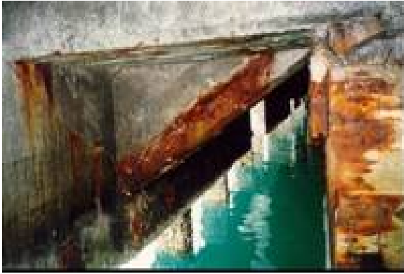
Figure 1-3: Corrosion damage on marine structure
