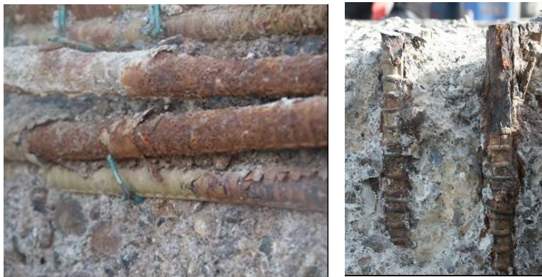
Figure 6-2: Illustration of the adverse corrosion protection performance of epoxy coated reinforcement in the vicinity of the saline waters of the Arabic or Persian Gulf under hot and humid environments.
