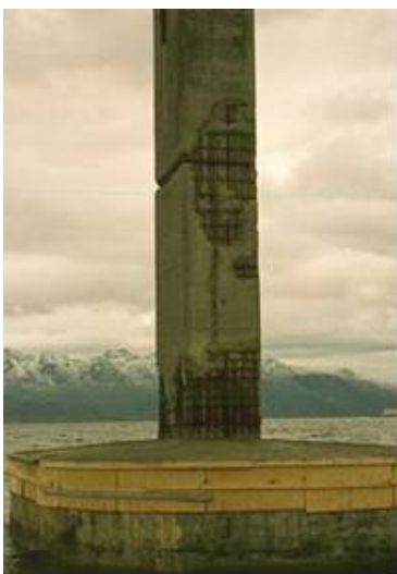
Figure 1-1: Corrosion damage on bridge pier.
