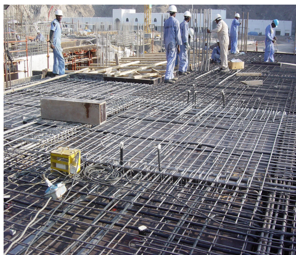
Figure 4-3: Combination of stainless steel reinforcement and ordinary black steel reinforcement. Only the deck part later to be exposed to a marine environment is reinforced with SSR. The remaining part of the deck, later to become part of the indoor structure, is reinforced with ordinary carbon steel reinforcement. No special precautions are needed where the two types of steel meet.
