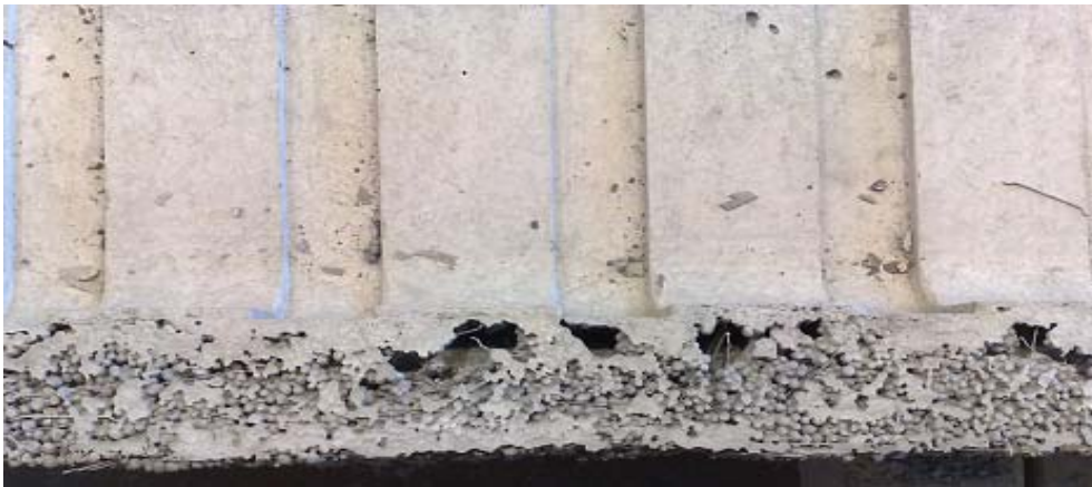
Figure 21 – Beam with separating concrete in the flange
