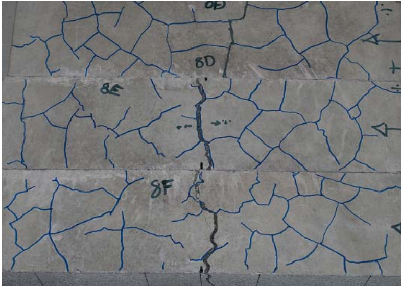
Figure 18 – Crack pattern in Standard test beams
