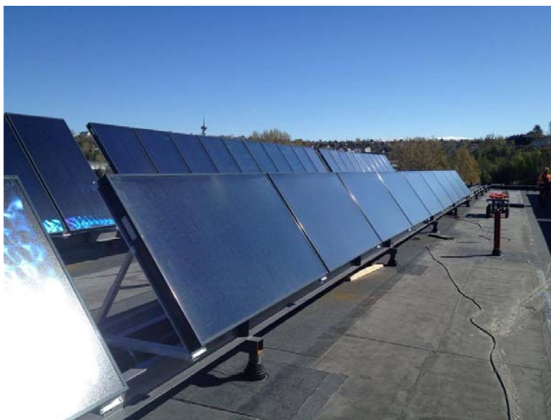
Figure 14 Solar thermal array at Scandic Hotel Lerkendal.
