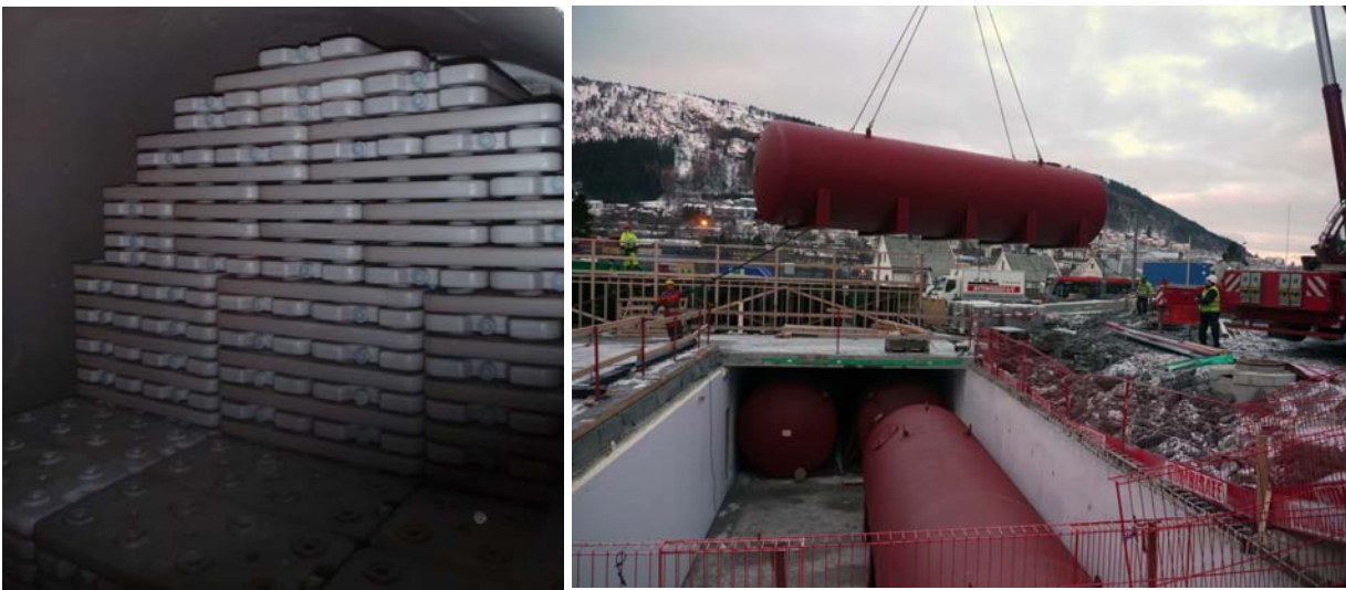
Figure 16 PCM elements inside the cold storage tanks (left) and cold storage tanks being placed underground at the Bergen University College (right) [27].
