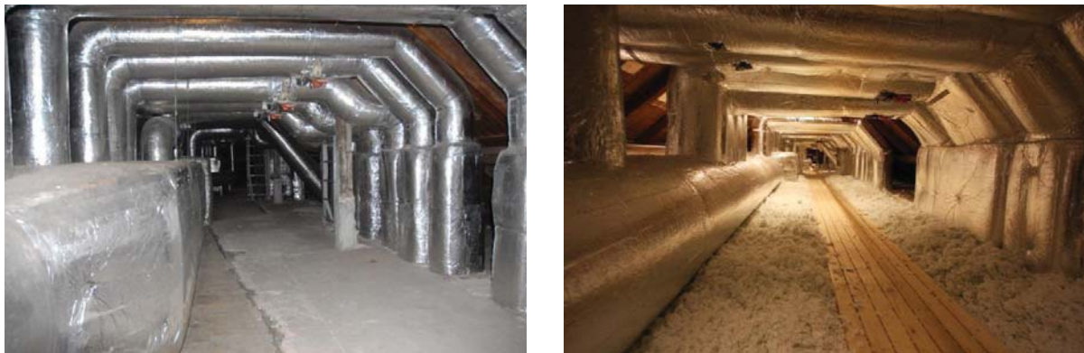
Figure 3 (a): Attic with ventilation ducts before additional insulation. (b): Attic with ducts after insulation. Photo: J. Seehusen, May 2012
